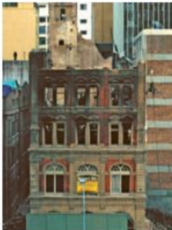
91 : The building damaged by fire in 1996.
