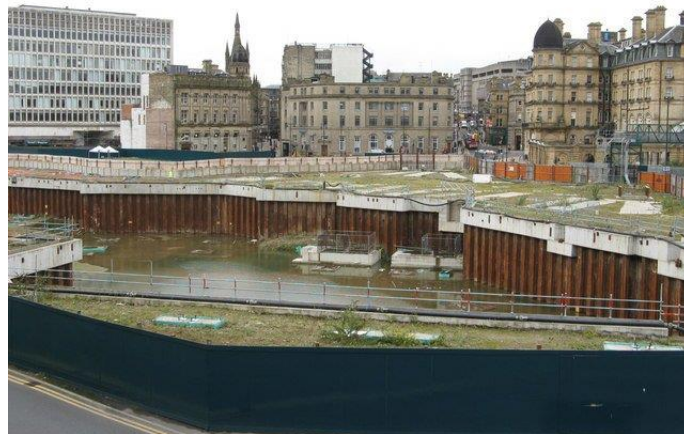
Figure 1: Bradford city centre hole (Source: The Construction Index, 2012)
