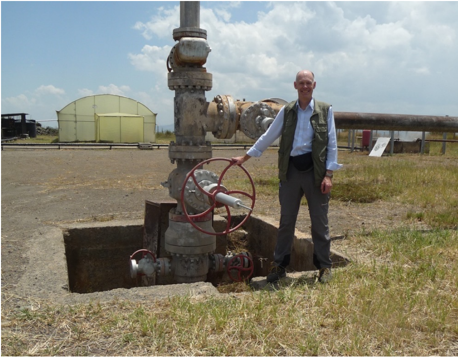
Figure 6. A typical production well at the Menengai Geothermal Field.
