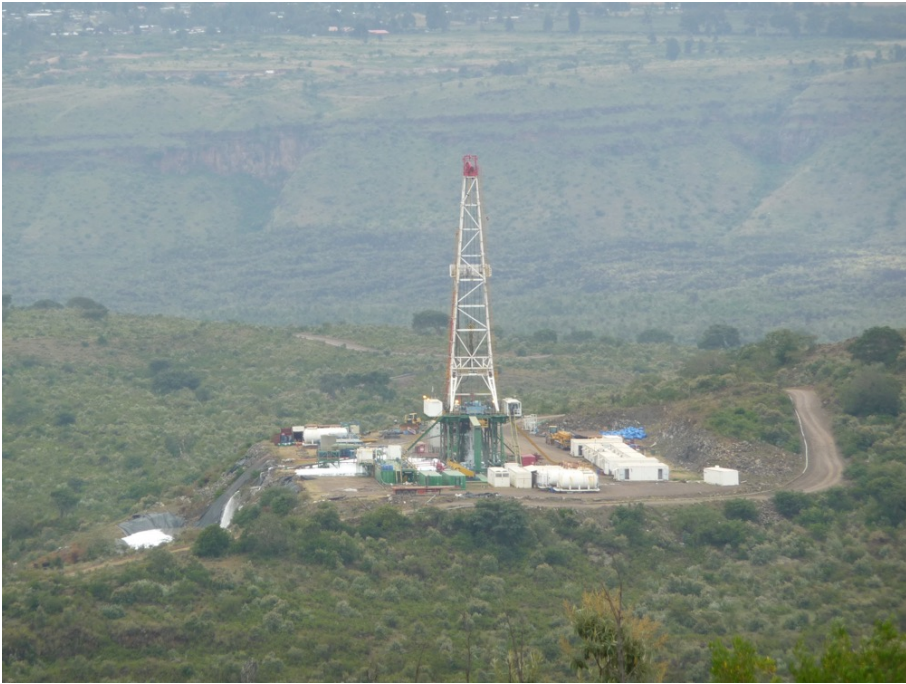
Figure 5. A large rig drilling a new borehole at the Menengai Geothermal Field. White containers on the right hand side give a sense of scale.
