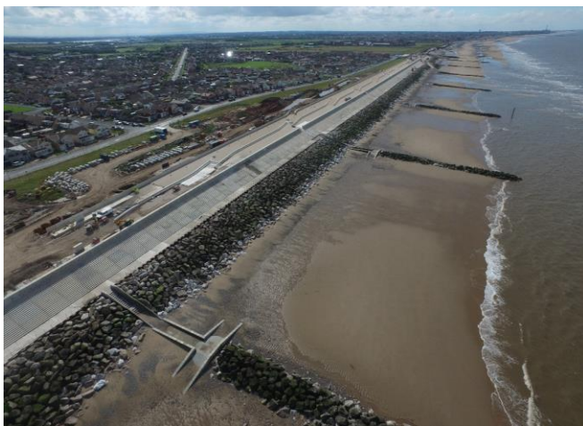
Figure 1. The Rossall scheme due to be completed in 2018. Drone photo provided by Balfour Beatty.
