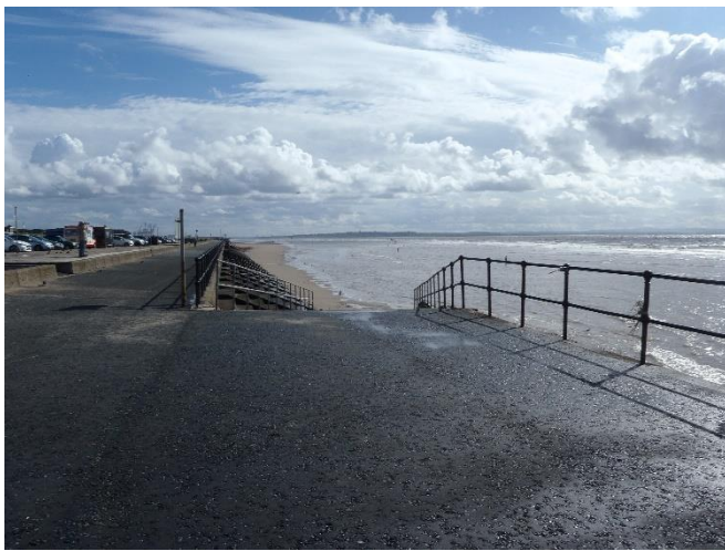
Figure 5. The northern end of Crosby sea wall where overtopping hazard to the carpark occurs.
