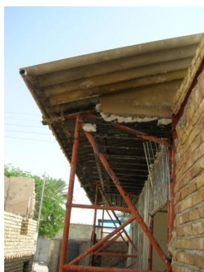
Figure 27: Difficulties in attaching new parts to the employed alien roof system in original PEHs
