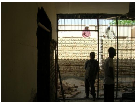
Figure 26: Workers are demolishing some parts of an original PEH due to heterogeneity of local materials and those applied in original PEHs
