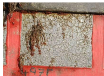
Figure 3:11: Cracking of biocidal polymers MESQ(I)25
