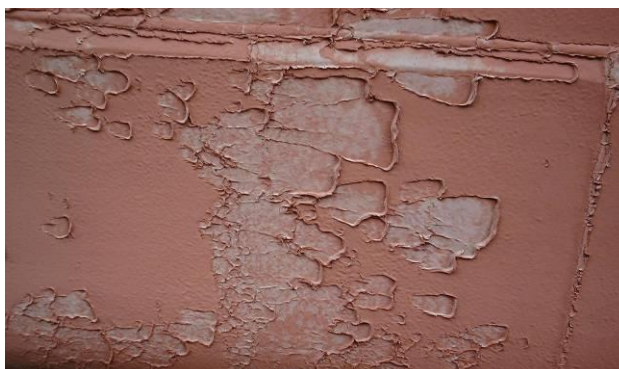
Figure 2:9: Example of 'cold flow' from the port side of a commercial vessel
