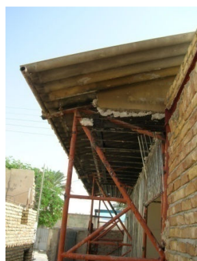
Fig. 19 Difficulties in attaching new parts to the employed alien roof system in original PEHs
