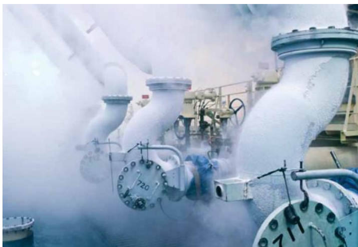
Figure 7.1: Vapour cloud resulting from condensing LNG.
