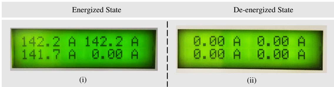
Figure 4-19. HMI of the MiCOM P122 IED on feeder 5
