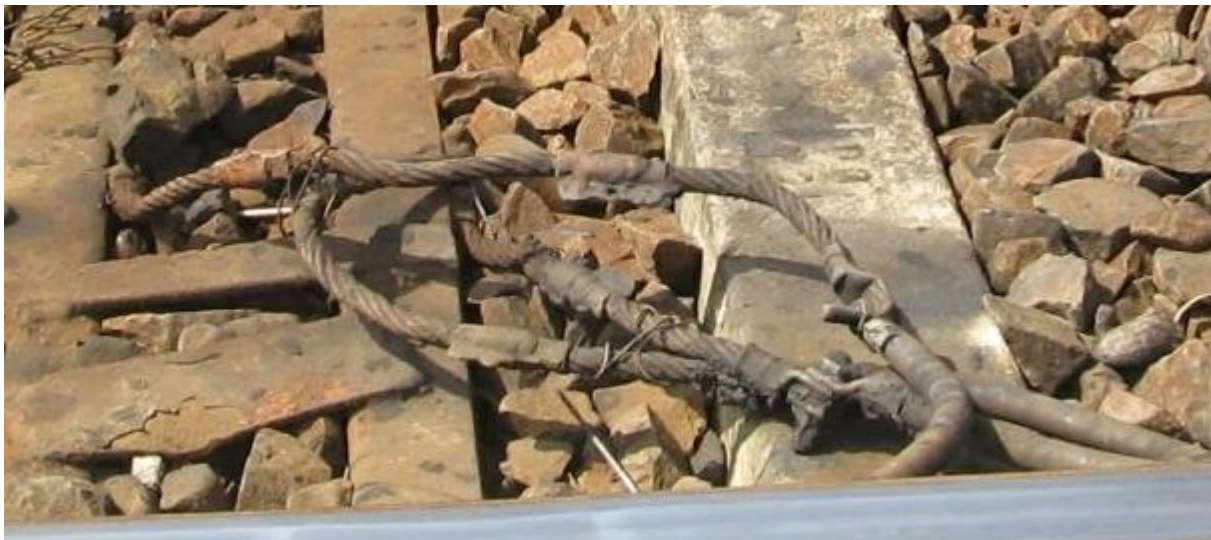
Figure-4.9 Traction Substation Negative Return Terminations.
