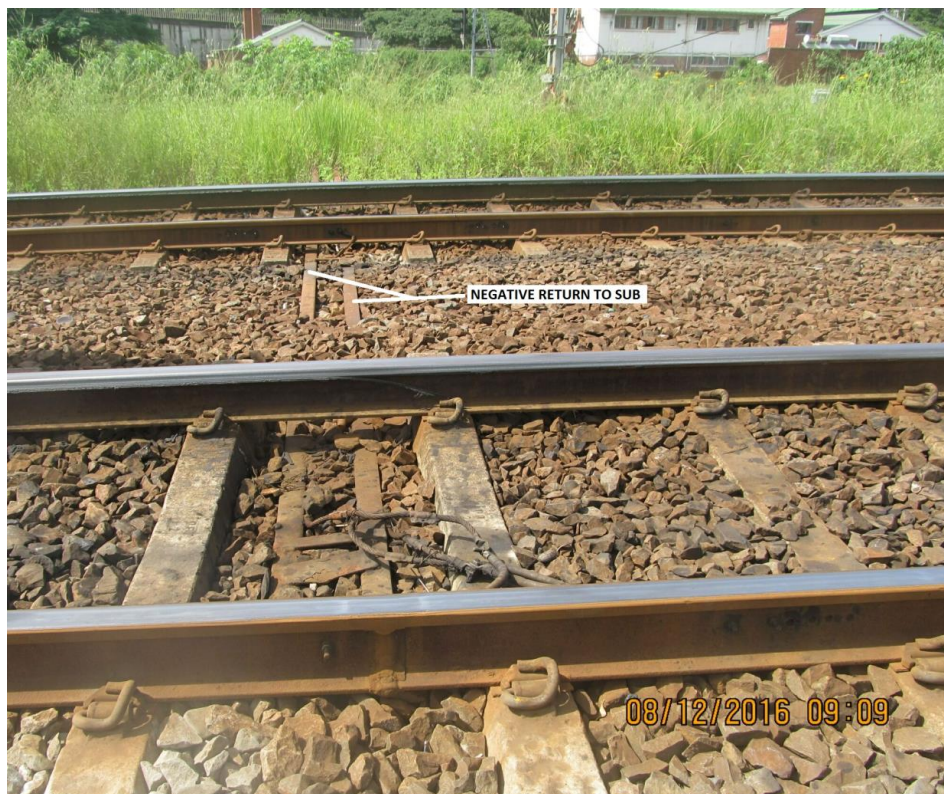
Figure-4.8 Bare Rail used as a Negative Return Conductor.
