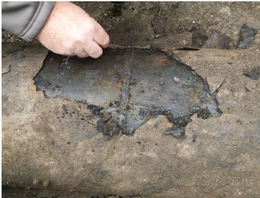
Figure-4.13 Coating Disbondment on a Petroleum Pipeline [48].
