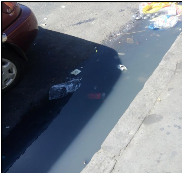
Image 12: Drainage system failure along road and pavement reserve (Source: Researcher, 2015) 16
