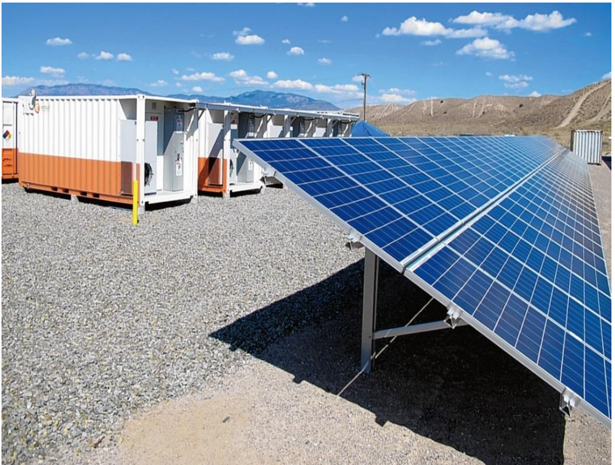
Figure 27: University New Mexico, USA, Ecoult/East Penn Manufacturing battery storage system
