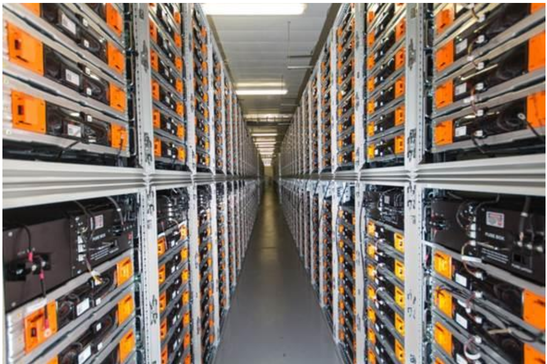
Figure 23: Tehachapi, California, United States, 32MWh Li-ion battery storage system [45]
