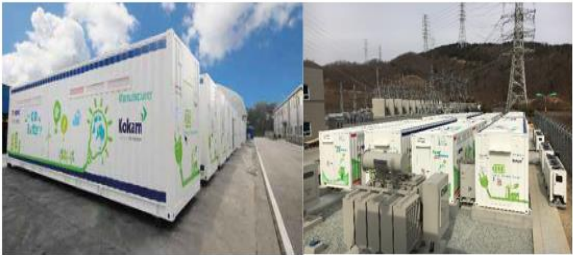
Figure 34: Gimje-si, South Korea. 24 MW Li-ion battery storage system KEPCO / Kokam [45], [50]
