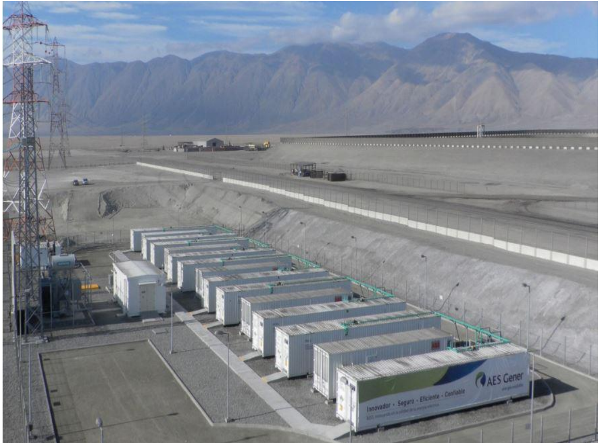
Figure 28: Mejillones, Antofagasta, Chile. 20MW Lithium ion battery storage system
