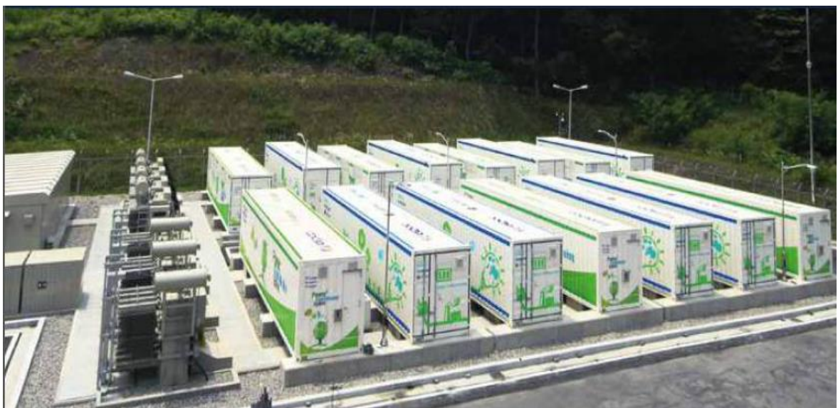
Figure 42: South Korea. West-Ansung (Seo-Anseong) Substation. 52 MW across 2 sites [50]
