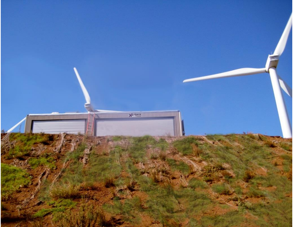
Figure 21:Maui, Hawaii, Lead acid battery system [45]
