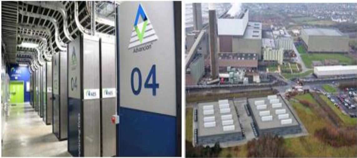
Figure 37: Northern Ireland, United Kingdom. 10 MW lithium ion batteries [45], [58]
