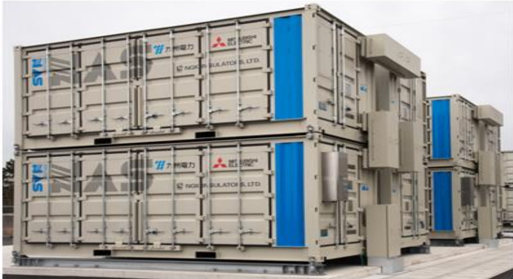
Figure 46: Buzen, Fukuoka Prefecture, Japan. 50 MW Sodium sulphur (NaS) battery system [55]
