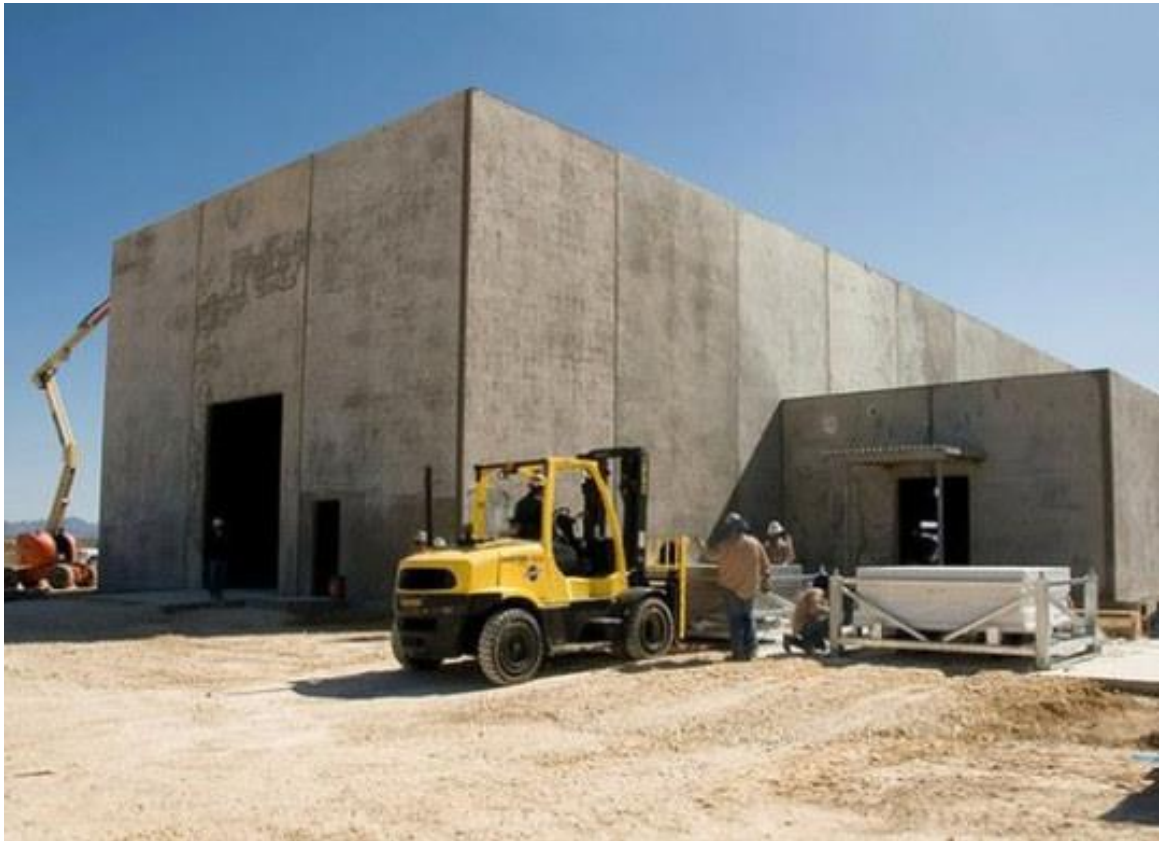
Figure 31: Presidio, Texas United States of America. 4MW Sodium Sulphur battery system [45]
