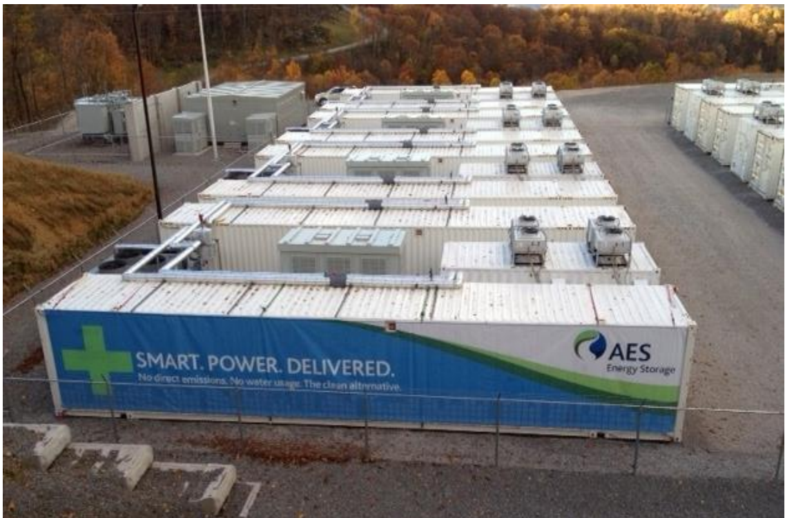
Figure 35: Elkins, Laurel Mountain Windfarm, West Virginia, USA. 32 MW lithium ion batteries [45]
