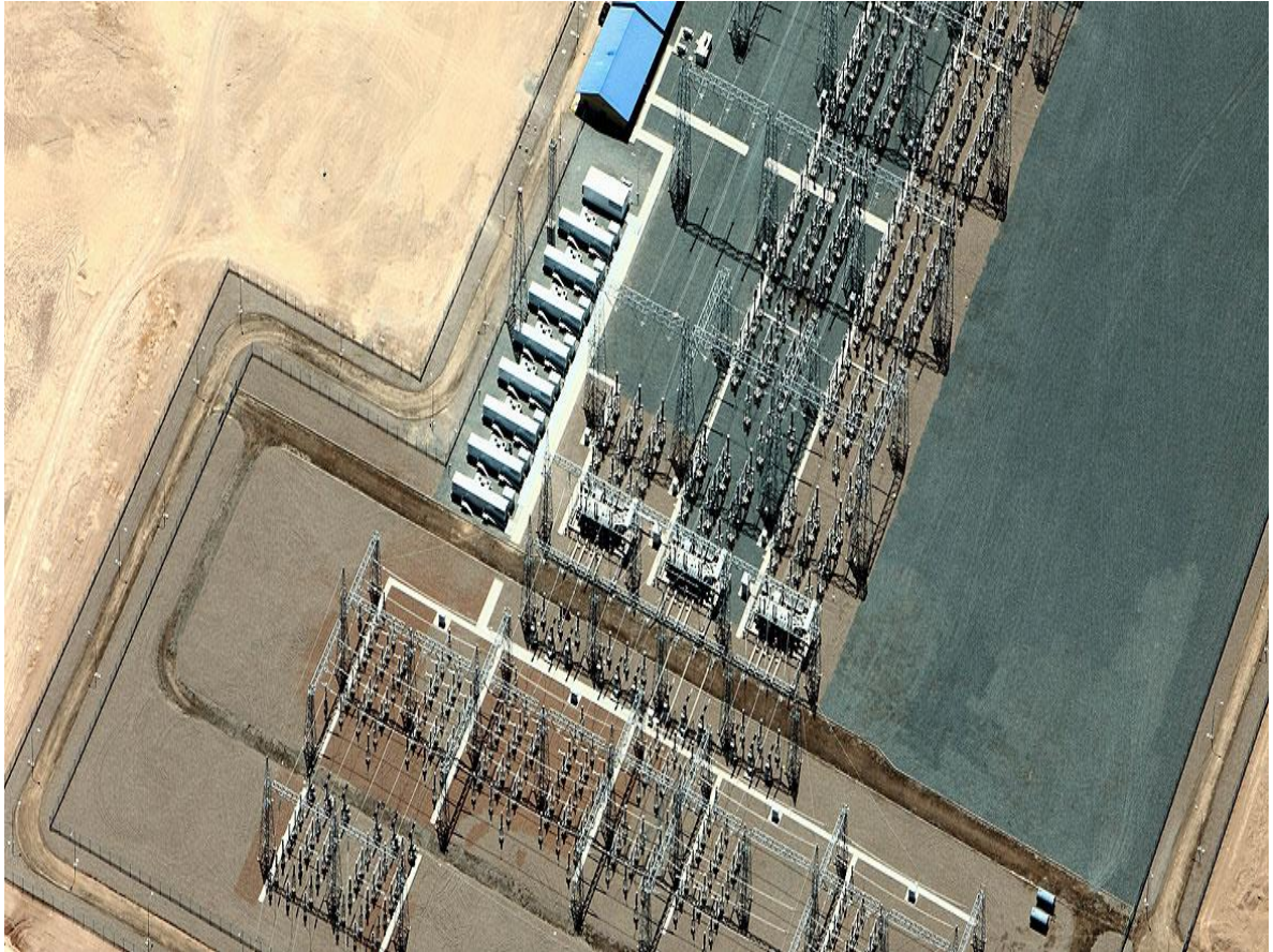
Figure 26: Copiapo, Atacama, Chile, 12MW lithium ion battery storage system [45]
