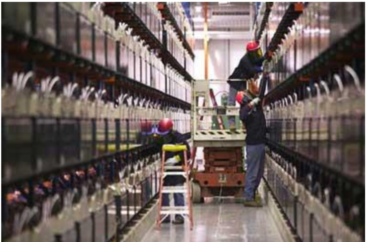
Figure 30: Fairbanks, Alaska United States of America. 27MW Ni-Cad battery storage system [45]
