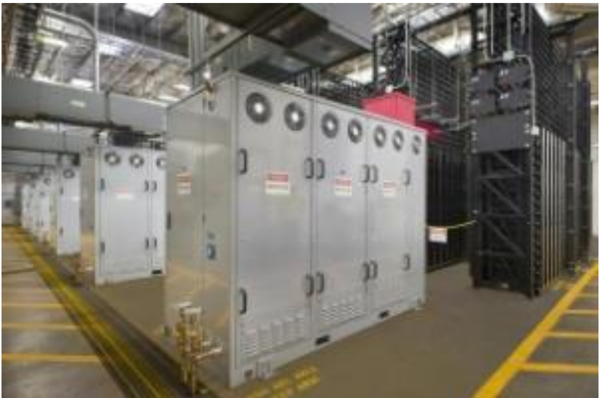
Figure 20: Kahuku, Hawaii Yunicos 15MW Lead Acid Battery Storage System [45]
