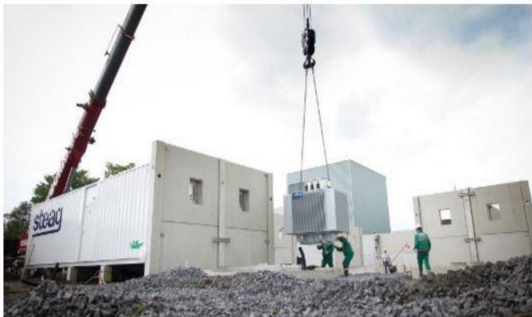
Figure 41: Lünen , North Rhine-Westphalia, Germany. 15 MW lithium-ion battery system
