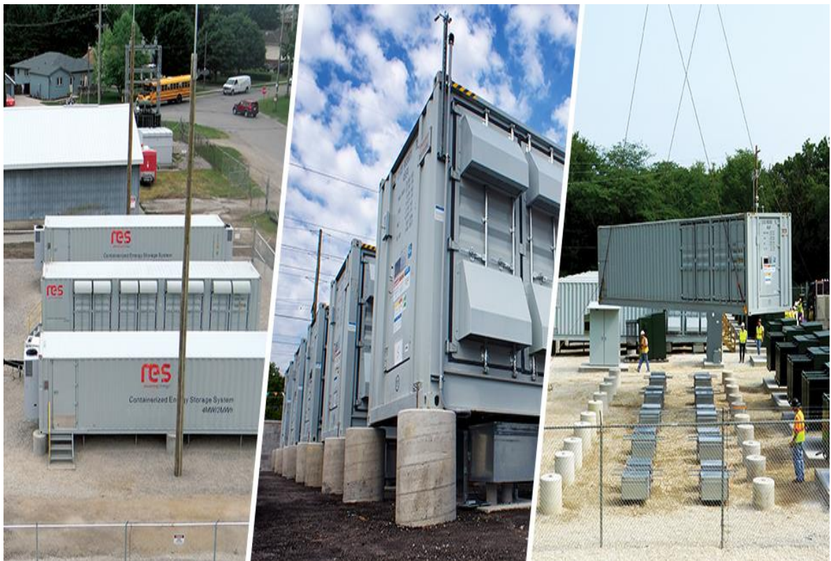
Figure 32: Illinios, USA, RES Americas 2x19.8 MW lithium iron phosphate batteries [45]
