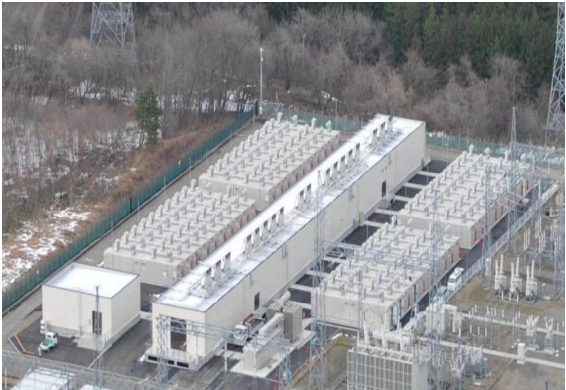
Figure 36: Sendia, Japan, Nishi-Sendai Substation. 40MW lithium-ion battery system [45]
