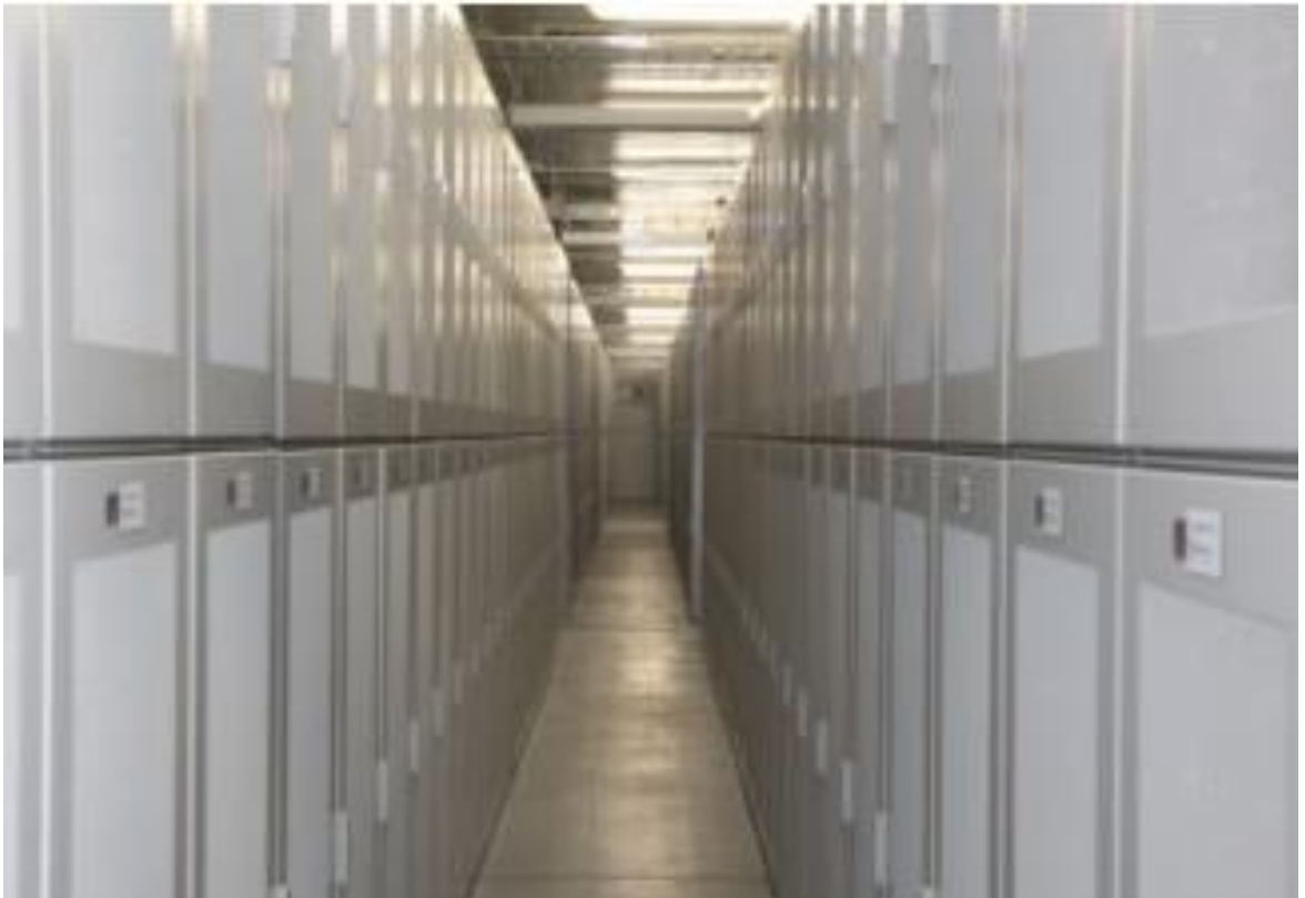
Figure 22: Tehachapi, California, United States, 32MWh Lithium-ion battery storage system [45]
