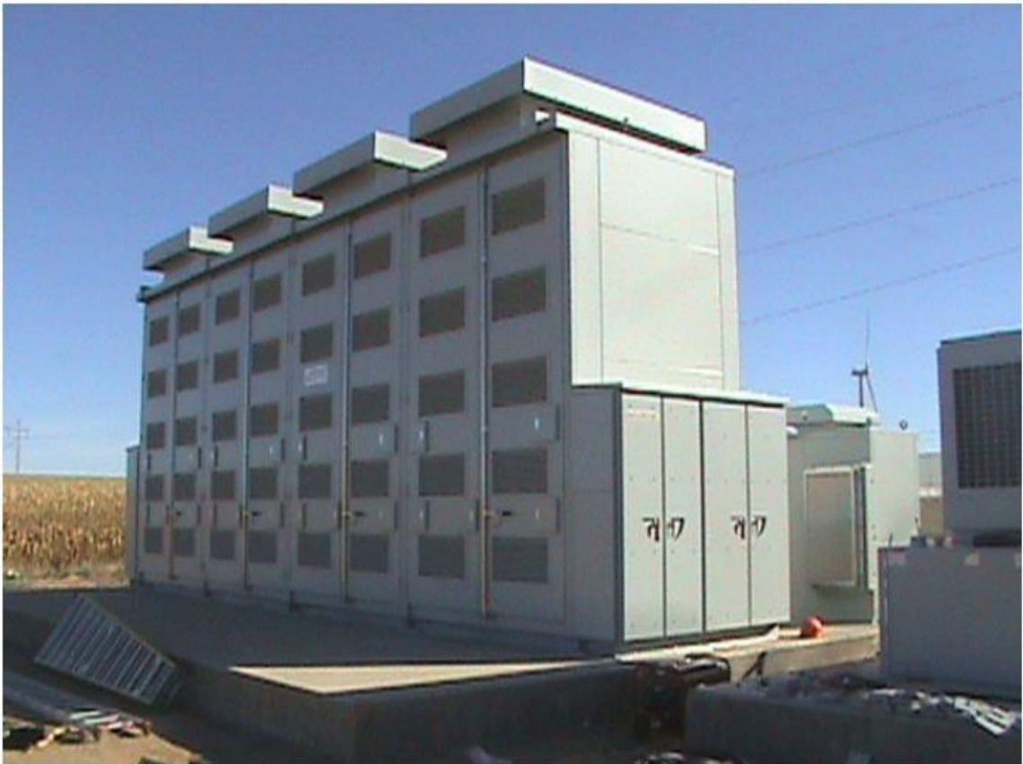
Figure 29: Luverne, Minnesota, United States, Sodium Sulphur battery storage system [45]
