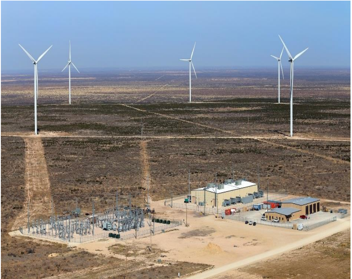
Figure 24: Goldsmith, Texas, United States. 36MW advanced lead acid battery system [45]
