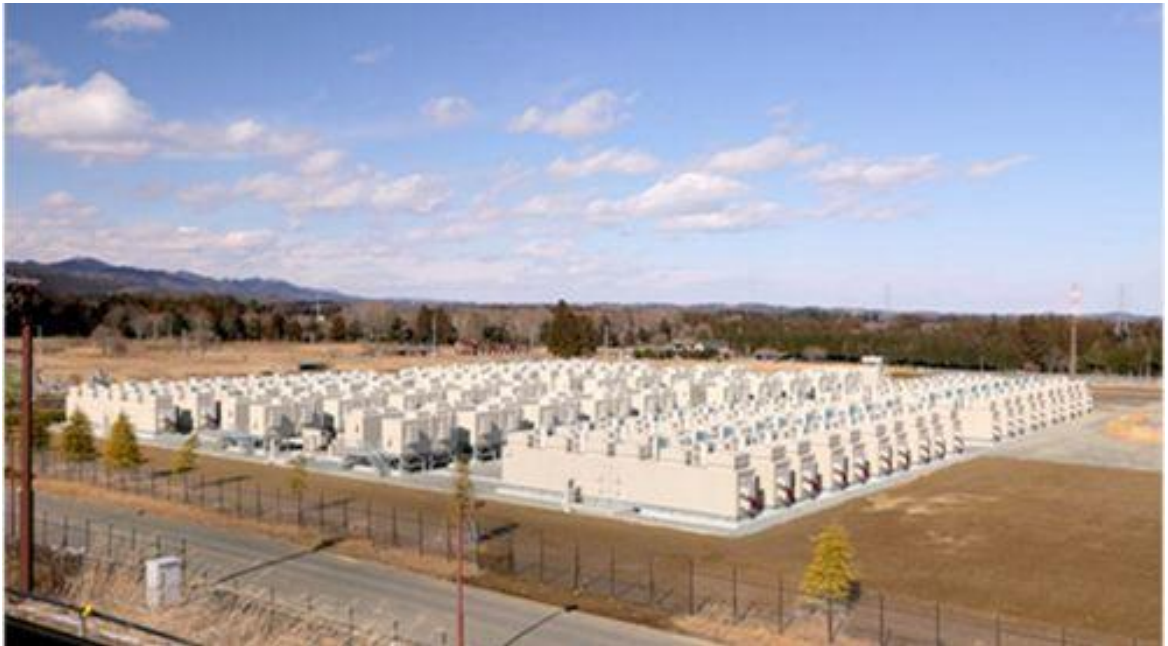
Figure 40: Minamisoma, Japan. 40 MW lithium ion battery system
