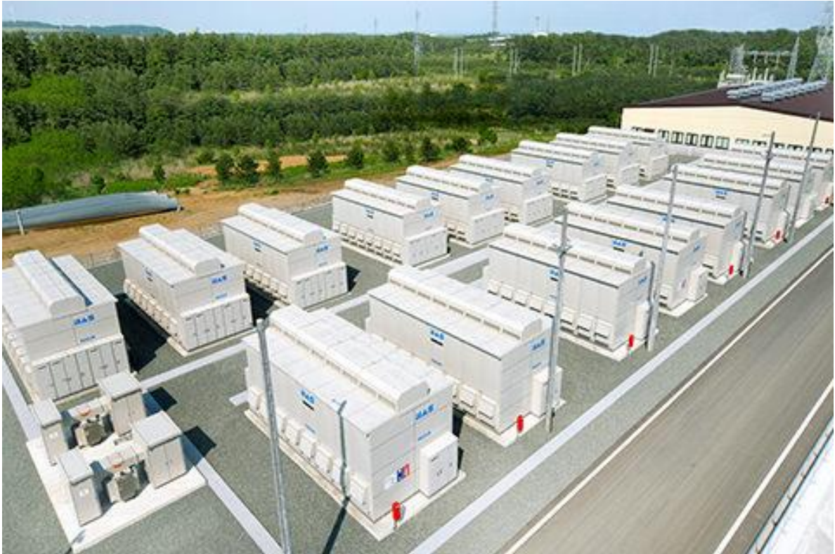
Figure 45: Rokkasho, Japan. Rokkasho Village Wind Farm using sodium sulphur (NAS) batteries [53]
