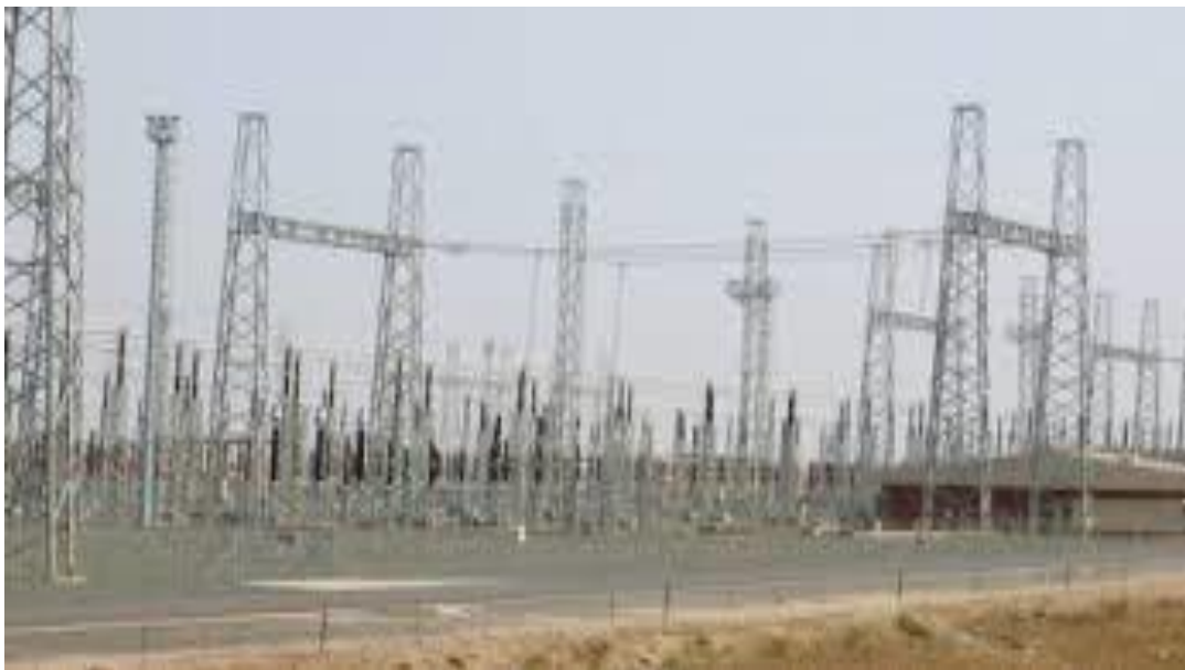
Figure 7.3: Kusile 400kV substation (Eskom)
