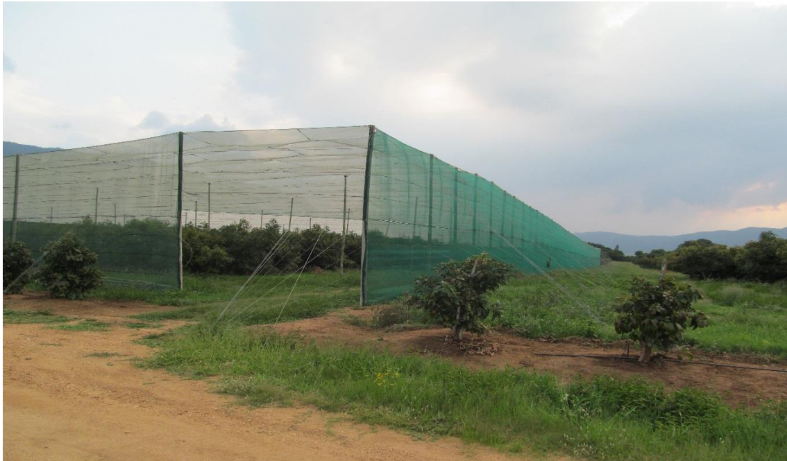
Figure 3.1 White shadenet structure over roof top with 40% green on the sides constructed at Mooketsi Valley
