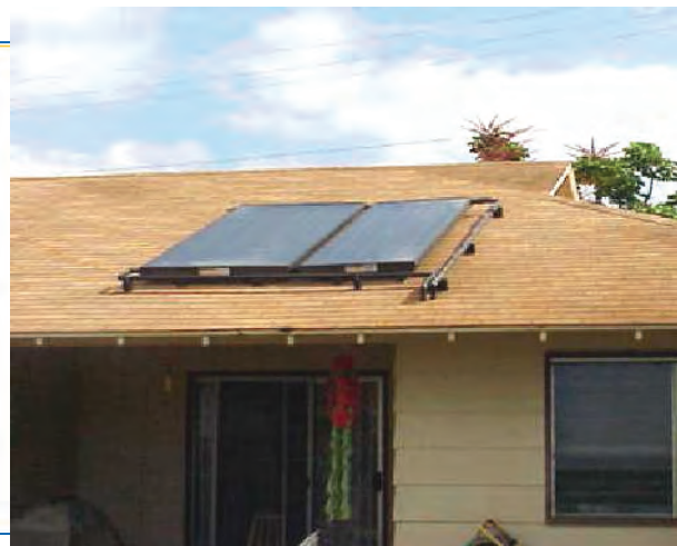
Figure 4: Flat-plate thermal solar collectors for providing hot water. (photo courtesy of DOE/NREL, Warren Gretz)
