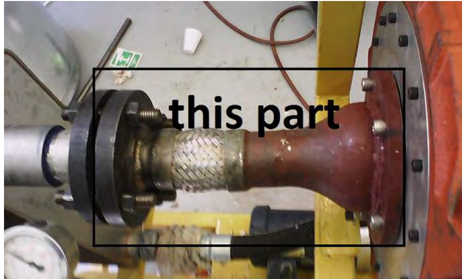
Figure 7.11: Defective turbine exhaust unit
