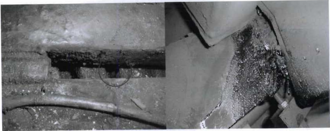
Figure 4-5: Area of extreme heating and bar damage
