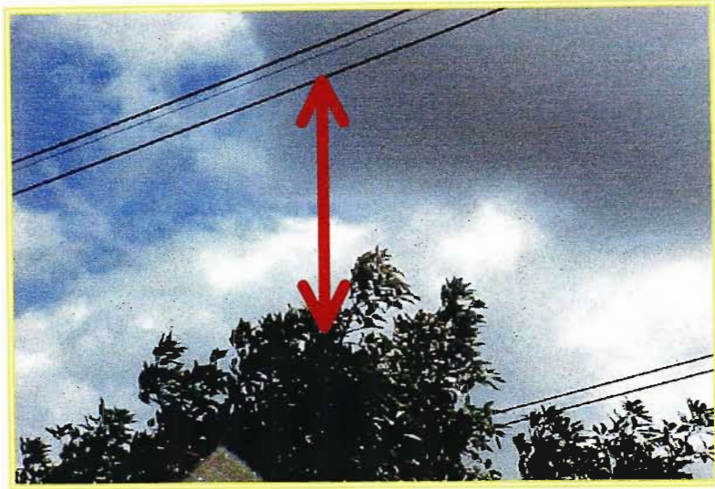
Figure 19. Photograph taken of the encroachment of trees under an overhead Transmission line (Photograph taken by C Chiloane, Eskom Transmission)
