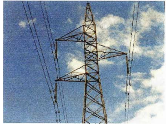
Figure 7. Delta Tower (275 kV)
