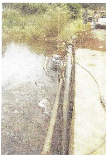
Figure 6.11 Abstraction of water from the Blyde River for the TGME mine at Pilgrim's Rest
