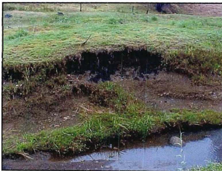
Figure 2.6. Mass bank failure.
