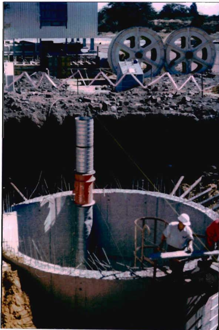
Figure 4.10 View westwards showing the sinking of the caisson of the Vertical Person's Shaft.
