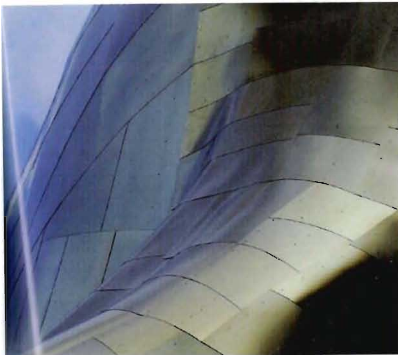
Figure 25_ Image showing the use of flat aluminium roof panel sheets in the EMP building to deal with the curved forms of the building. (Bruce. 2000: 29)
