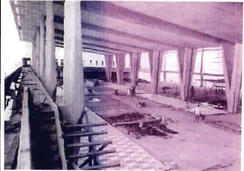
Figure 5.6_Image showing the reinforced concrete V-columns and concrete roof under construction in 1962. (Wale. 1962: 5)
