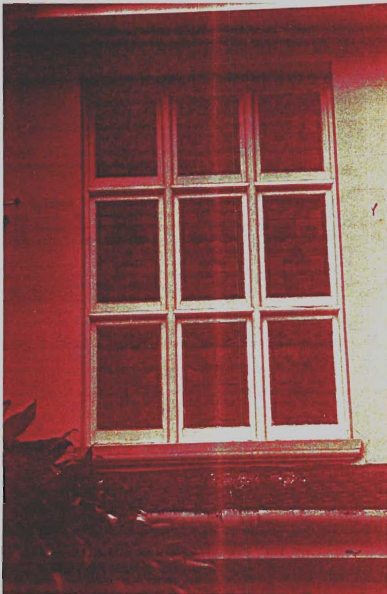
Staircase (demolished) window
