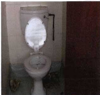
Plate 7: Water borne flush toilet
