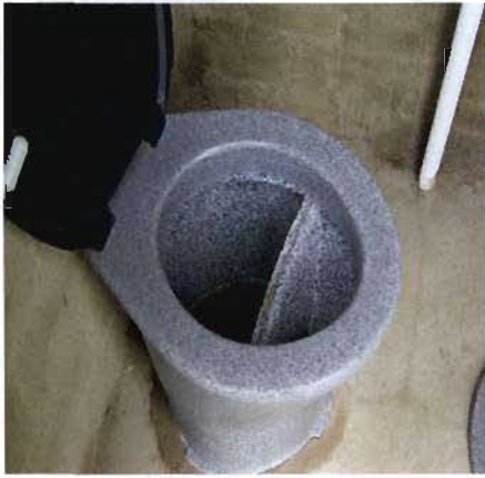
Plate 5: Urine diverting toilet
