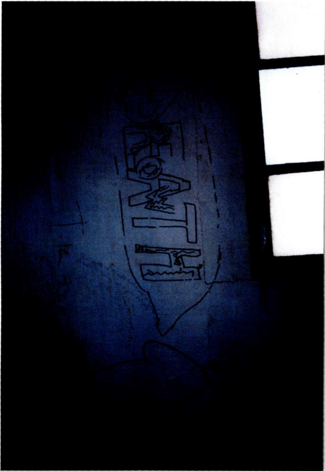
Picture 4: Graffiti in an Umzamo high school classroom wall
