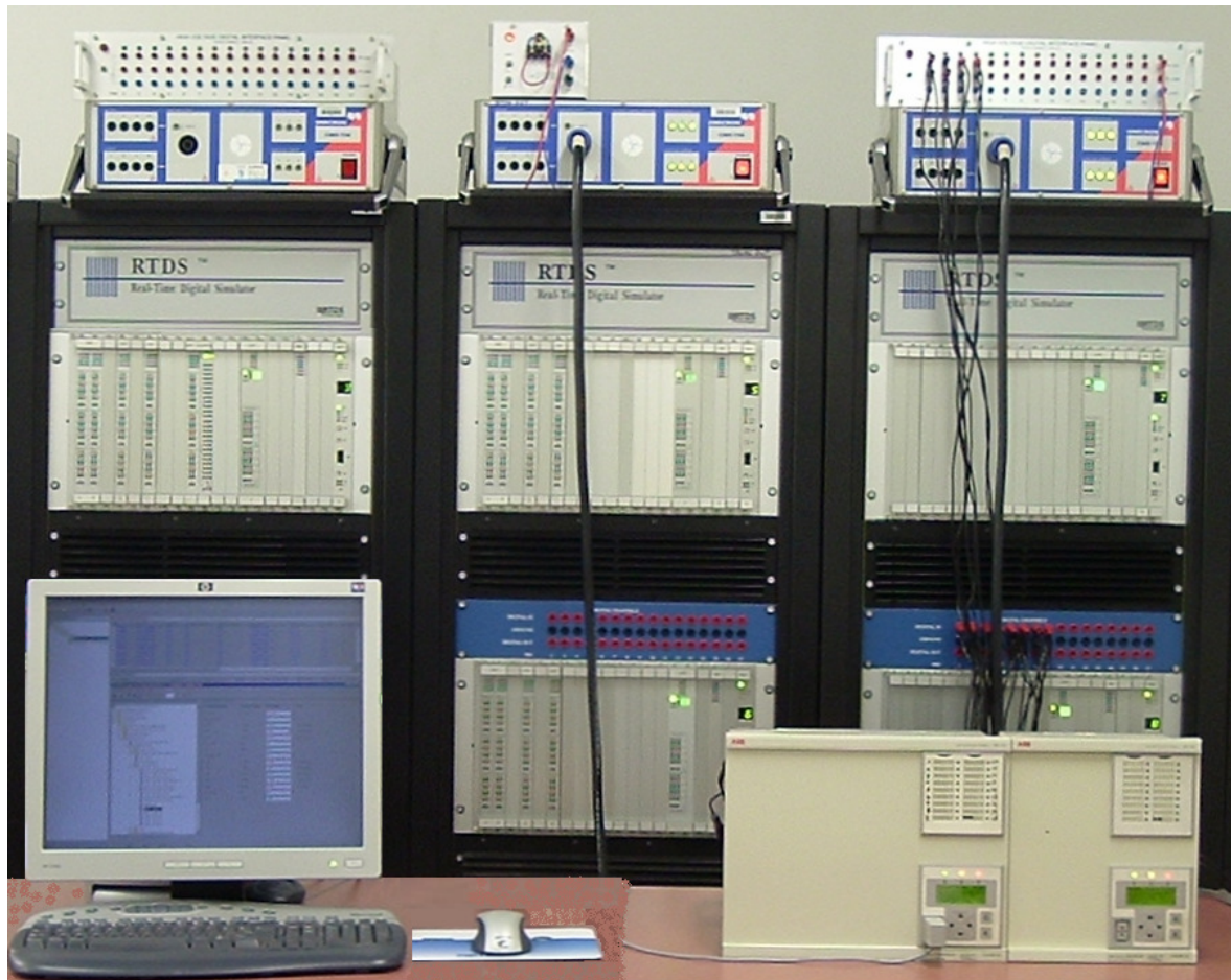
Figure A1: Hardware-in-loop testing of the REL531 relays using the RTDS.
