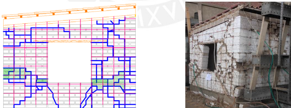
Figure 8. Sketch of damage pattern and general view of the model after second ( D_0 = 130 mm) test
