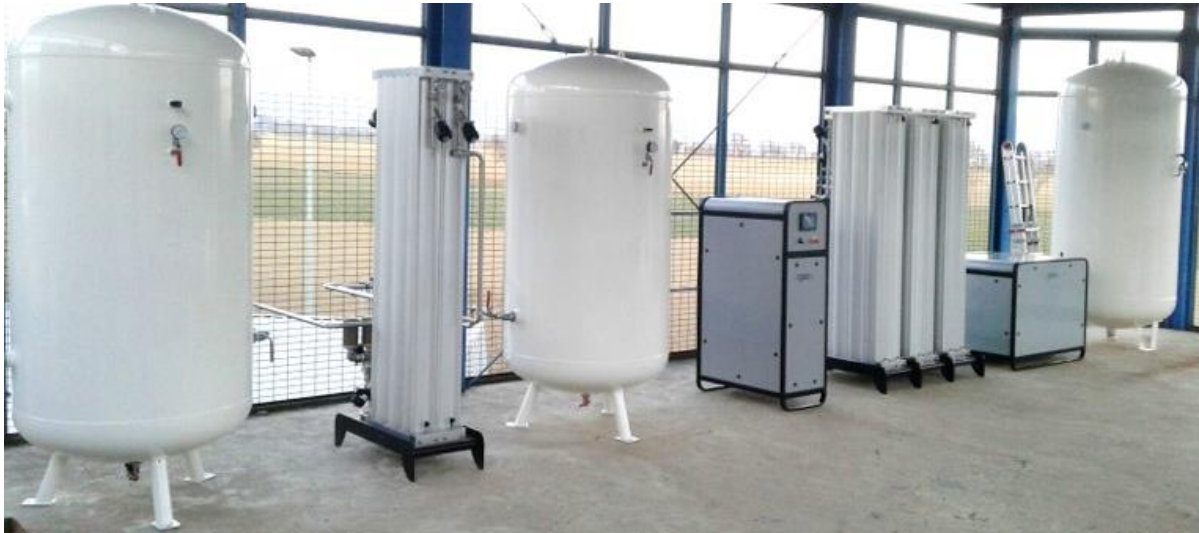
Figure 37: Picture the VPSA industrial plant for CO 2 capture and storage.
