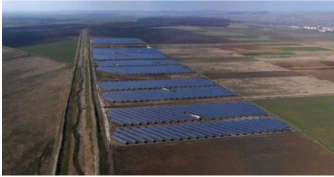
(a) Vanju-Mare PV plant image [61]
