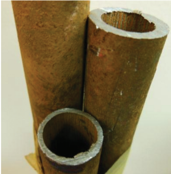
Figure 4: Section of the tube with severe uniform corrosion and wall thickness reduction.
