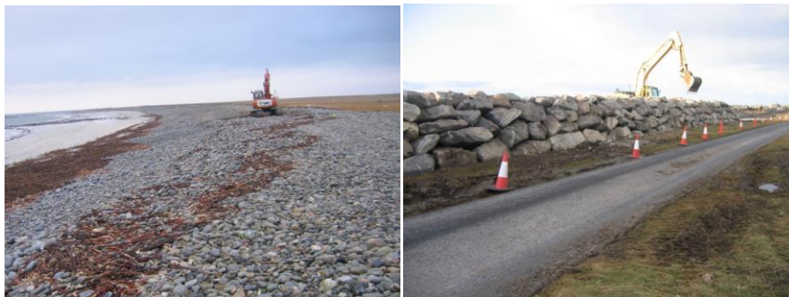
Figure 2. Coastal protection scheme at Stoneybridge, South Uist, showing reconstruction of the shingle ridge damaged during the 2005 storm (left) and rock armour (right)
