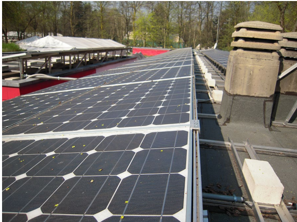
Fig. 23 Photovoltaic panels on the roofing of Circolo Magnolia (Milan, IT): because of a non optimal performance and placement, the project was primarily meant for marketing (picture of the authors)
