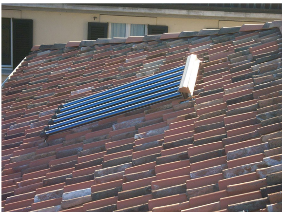
Fig. 25 Solar thermal panel on the roofing: regulatory requirement for the production of hot water (picture by authors)
