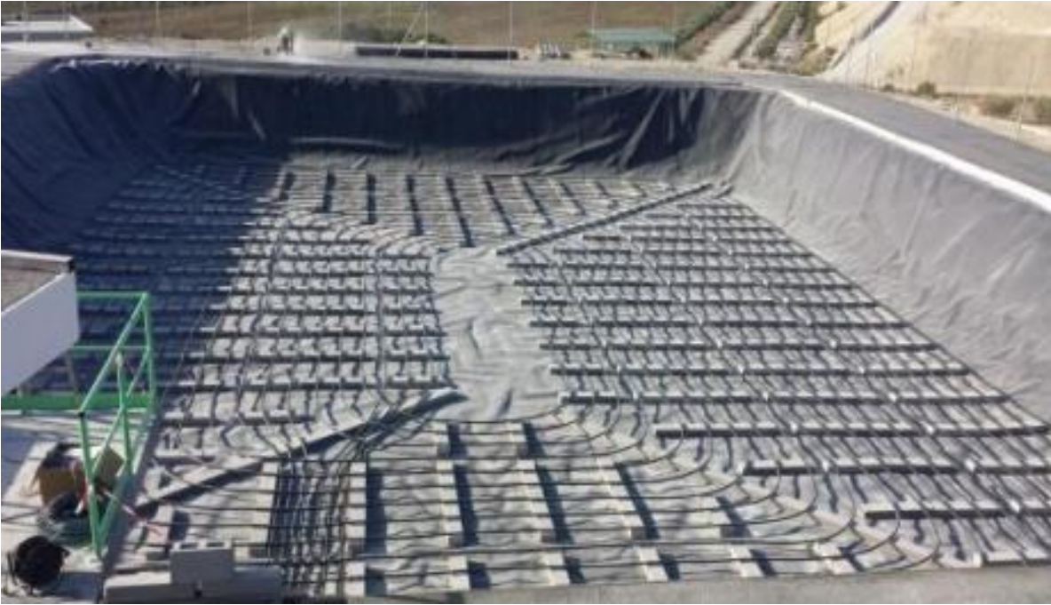
Figure 92. Final location of the heat exchanger
