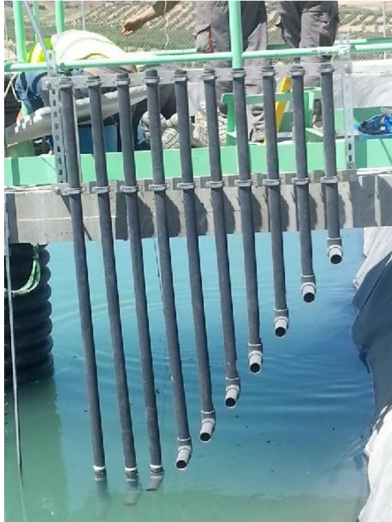
Figure 78. Pipe system to add acid in the system at different heights
