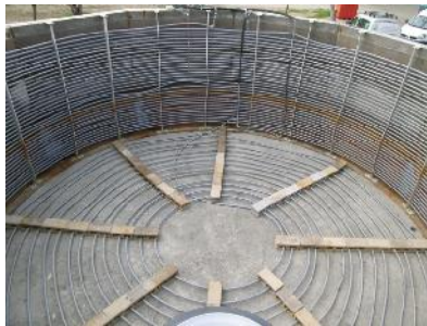
Figure 16. Lateral and bottom heat exchangers installed in solar pond Martorell
