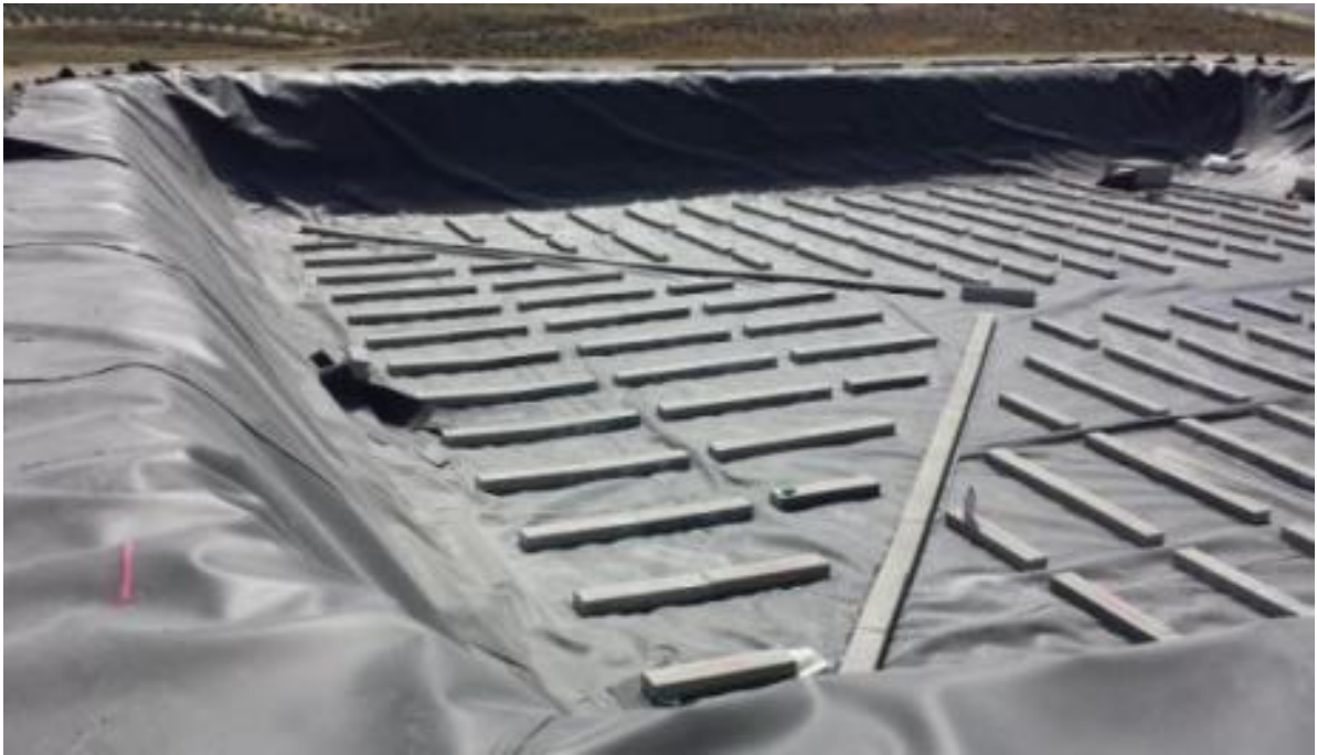
Figure 91. Structure of the concrete blocks in the bottom of the solar pond
