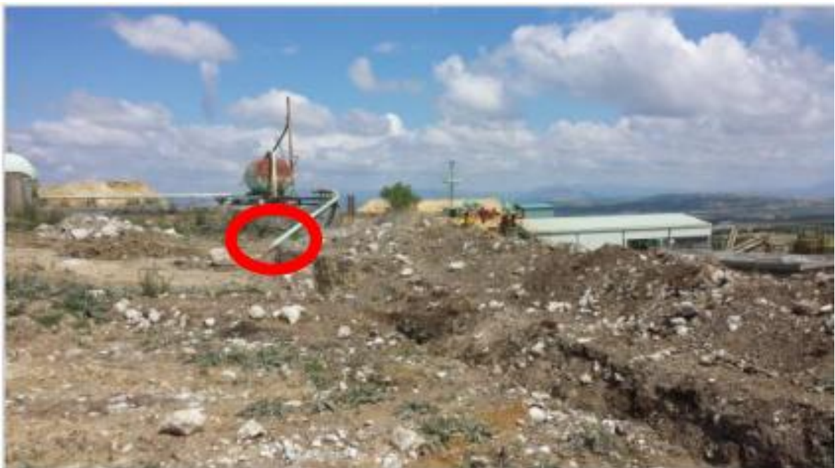
Figure 45. Initial location of the freshwater pipes in Solvay Minerales facilities
