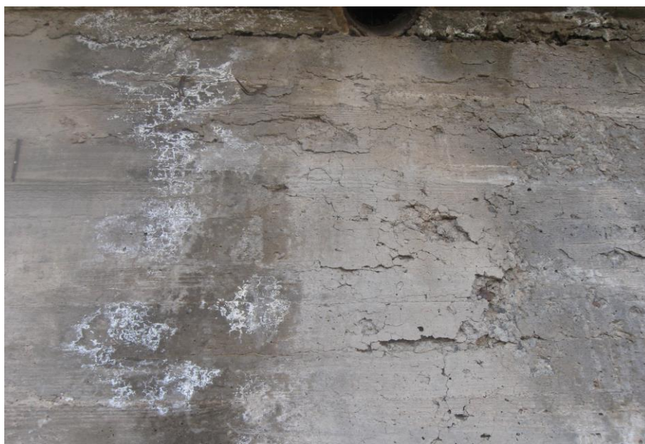
Figure 1.2 The cracked surface of reinforced concrete in a three span bridge slab in south of Kerman (Constructed in 1998)
