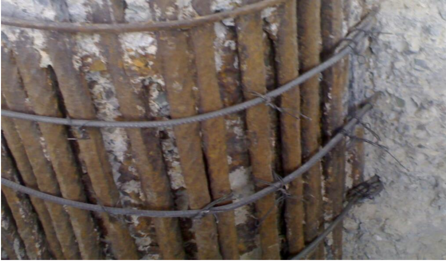
Figure 1.1 The corroded reinforcement sections of a three span bridge pile in south of Kerman (Constructed in 1998)
