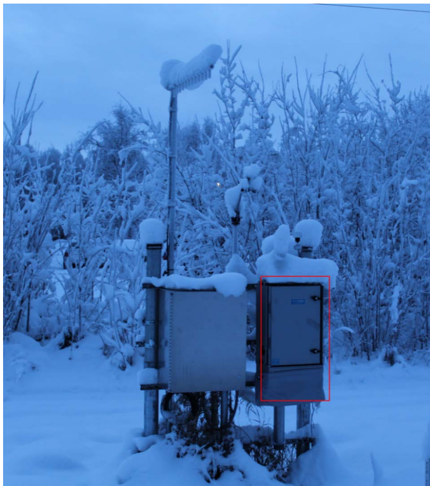
Figure 3.3 RWIS site equipped with AQM60 air quality monitor (rectangular box outlined in red) with other road weather monitoring devices
