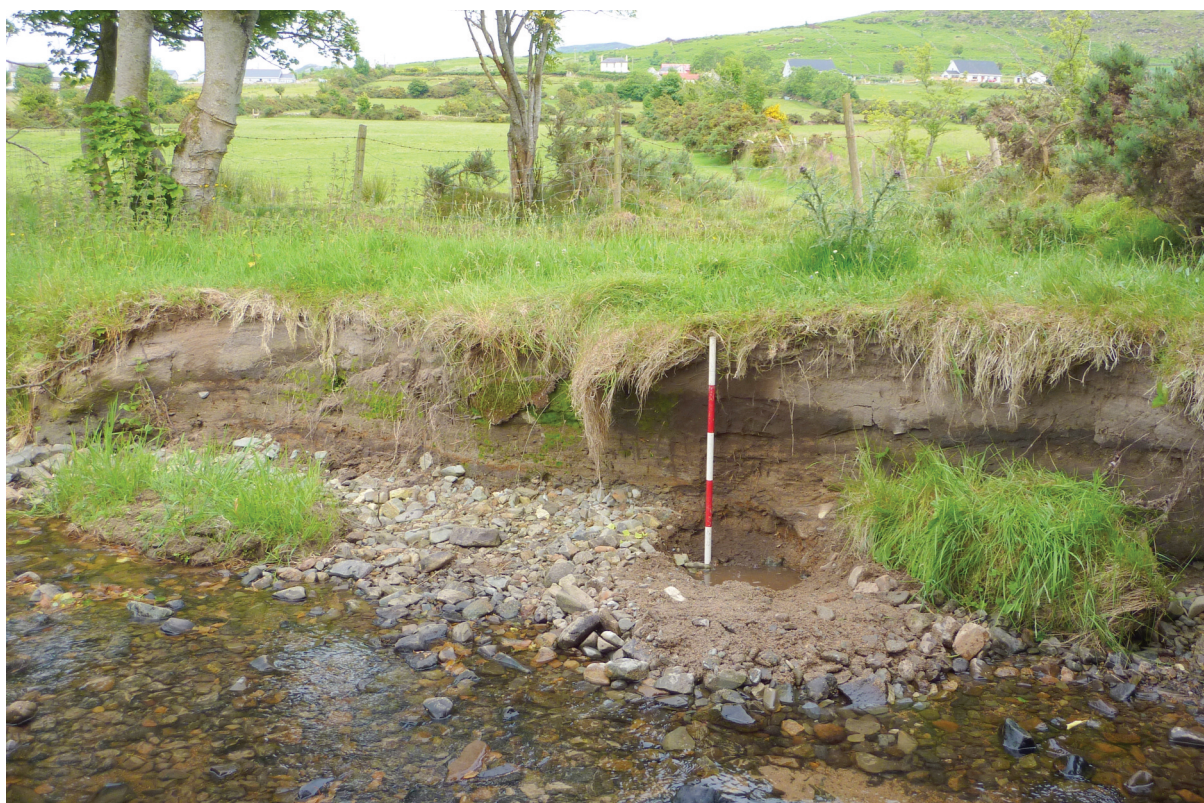
Fig. 4—Collapsed bank of river at site B. Section B is marked by the 1m ranging pole.
