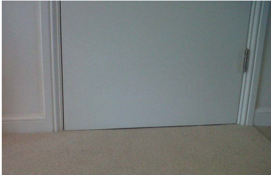
Figure 7.15. Insufficient air transfer opening between rooms.
