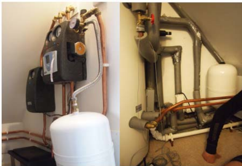
Figure 7.13. Uninsulated and poorly insulated pipework in the plant room.
