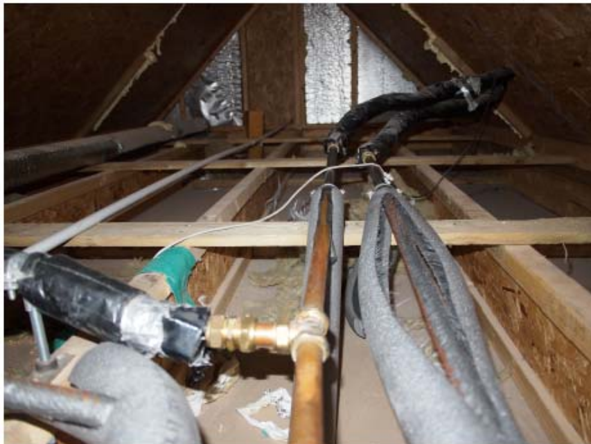
Figure 7.12. Solar system pipework in the attic of the Glasgow house showing poor specification and poorly applied thermal insulation. Much of the insulation was found to have melted and fallen away from the pipes.
