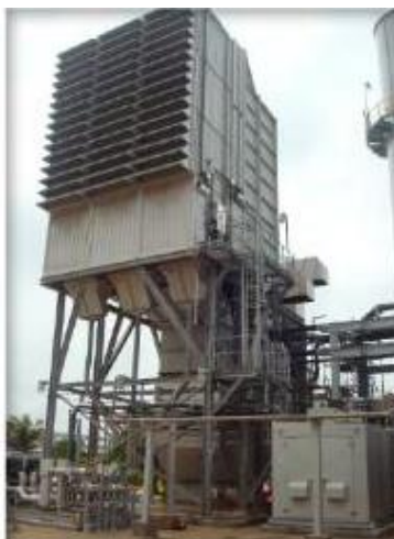
Figure 16: Inlet Air Filter House (Courtesy: CAMFIL)
