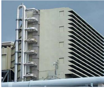
Figure 17: Inlet Air Chilling System Header (Courtesy of BHGE)
