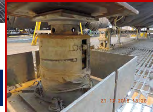
Friction plate pipe support with spring hanger base for main suction & discharge headers
