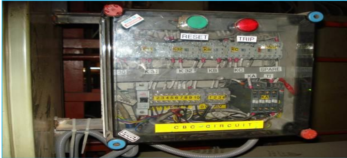
Fig 5.14. Photograph of Automatic protection module
