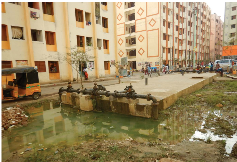
Figure 2: Housing built on marshy land is usually water-clogged which could have health implications in the long term
