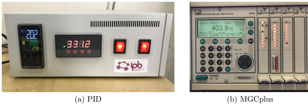
Figure 4.12: Heating and Monitoring System.
