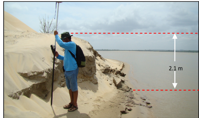
Figure 3. The banks of the mid-channel bar (study area) are associated with highly erodible unconsolidated deposits.
