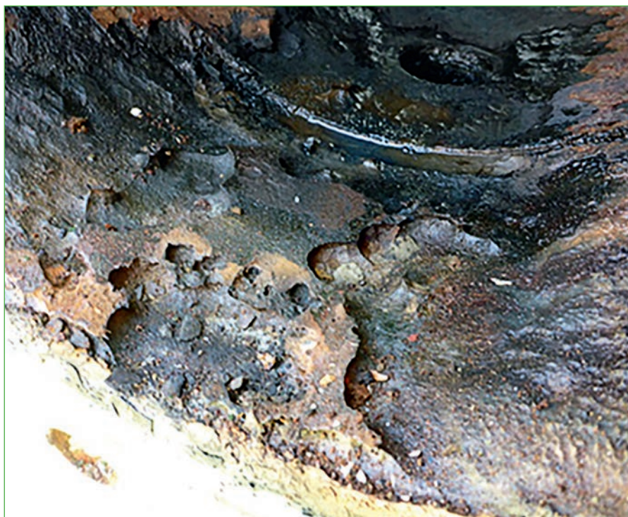
Figure 1 Microbiologically influenced corrosion of crude line to cargo storage in a Floating, Production, Storage and Offloading vessel (FPSO). Reproduced with permission from Machuca and Polomka (2018), Microbiology Australia 39 (3), 165-169.
