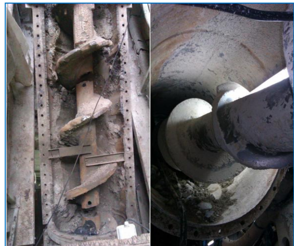
Fig. 9 Excessive wear on the screw conveyor of EPB-TBM
