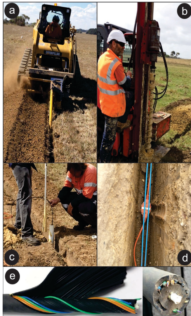
Figure 1. Experimental setup. Photos show a) the trencher digging the trench, b) boring for the 4 meters deep PVC cased bores to install geophones, c) the installation of a geophone in a bore and the geophone cables and d) blue iDAS fibre-optic cables laying at the bottom of each trench, and e) Helically wound cable buried in Line 5 trench for direct comparison (after Hornman et al. , 2013)
