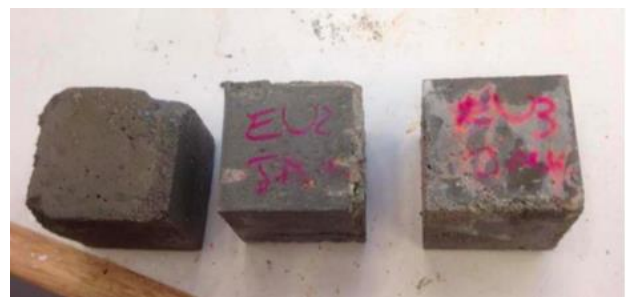
Figure 7. Visual Observation of Efflorescence on Unground Eraring Specimens for Each Design Mix.
