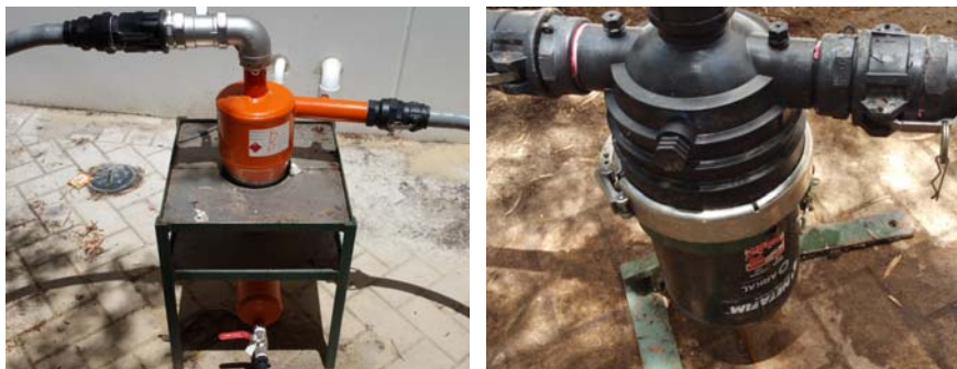
Figure 3.8 Hydrocyclons and filters.
