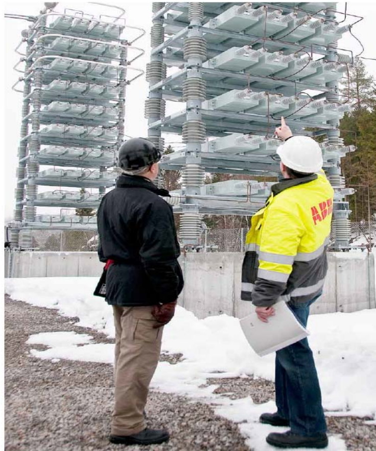
Fig. 4. 17 420 kV capacitor installation in Norway supplied by ABB [71]
