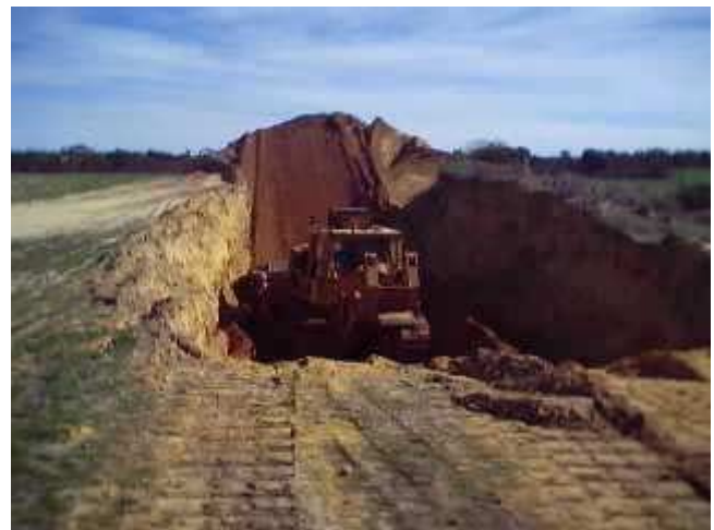
Figure 1. Excavation of the Hyden fault scarp using a D9 earthmover. The left-hand wall was kept near vertical so as to simplify geological mapping of the fault structures.
