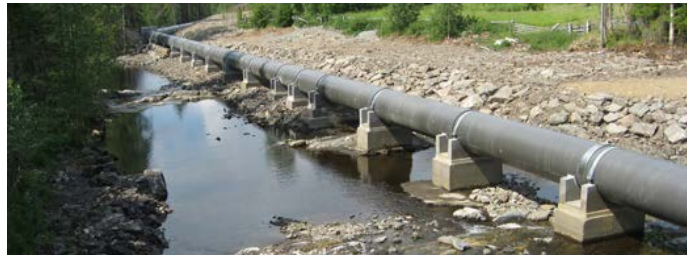
Fig. 4. A typical above-ground pipeline
